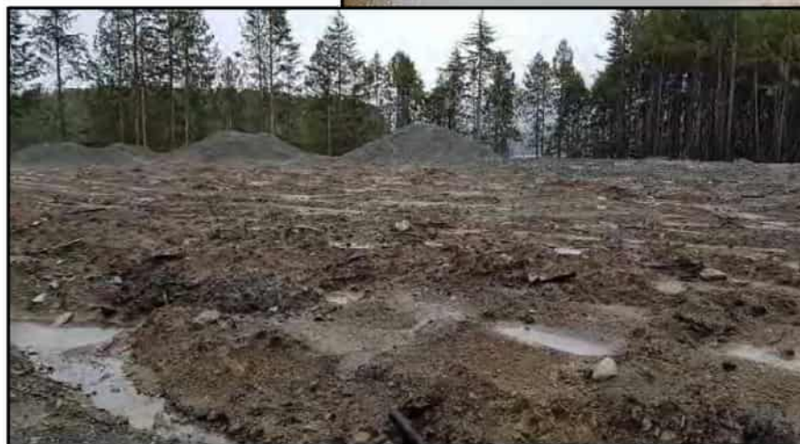
Photo 9: 2017 Image of cleared and grubbed section of site in northern half of property. Portion of foreshore buffer area cleared during tree removal.
