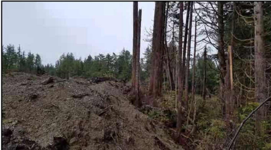
Photo 11: Stockpiled soil burying the base of some trees in 30m foreshore DPA needs to be removed.
