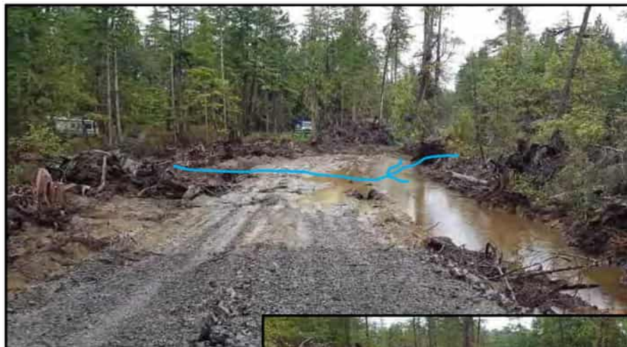
Photo 7: View on opposite side of road alignment. Pondered water along road at upper end of the Middle Stream side channel; Southern half of property.
